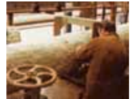
High temperature pipework
